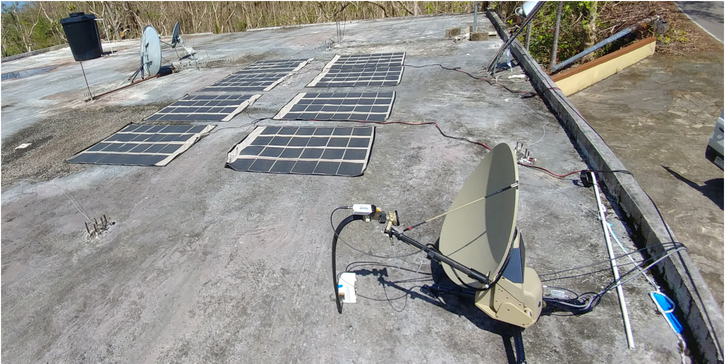
Figure 1 - Solar Stik System Powering Satellite Data Terminal on Puerto Rican Rooftop
