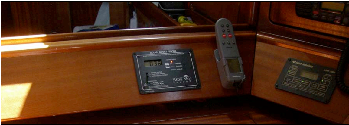
SOLAR BOOST™ CHARGE CONTROL INSTALLED
