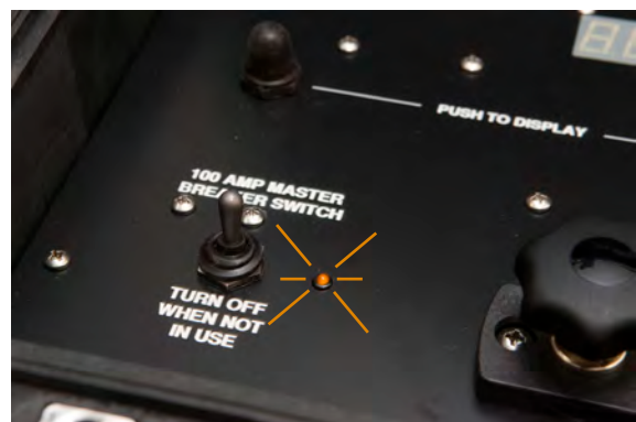
Figure 11 - 100 Amp Master Breaker Switch
